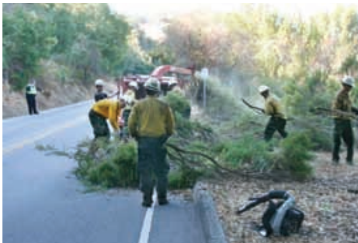
Clearing: Workers remove brush in the Los Trancos Water District. The district may be disbanded under a new state law if the state finds the district wasteful.
